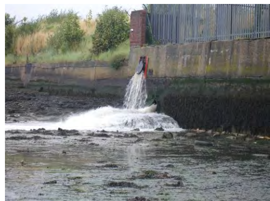
12: Woolston STW storm overflow
