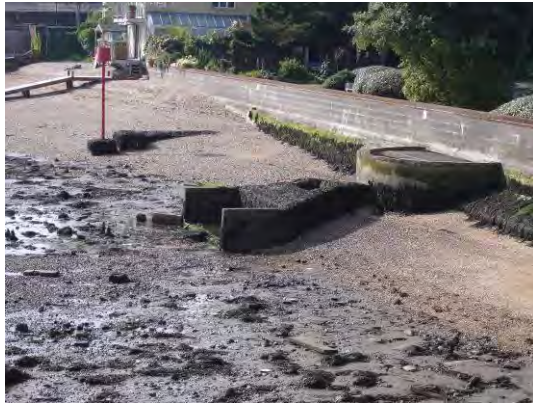
1: Alexandra Rd CSO outfall, Hythe
