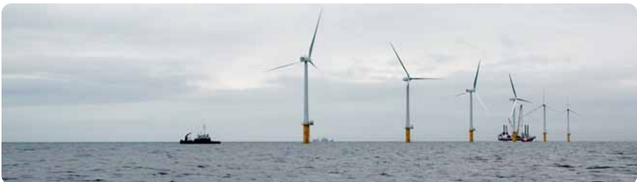
Left and Below: Wind farm under construction at North Hoyle, off the North Wales coast
