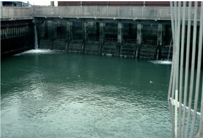
Figure 2 CW intakes (Heysham Power Station)
