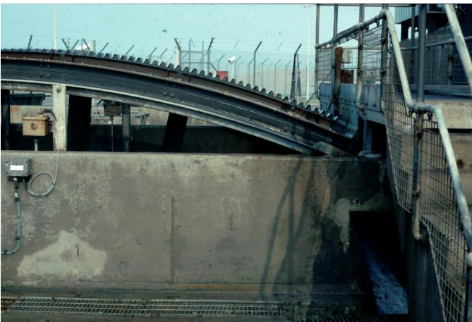
Figure 3 Drum screens showing back-wash culvert (lower left corner) (Torness Power Station)
